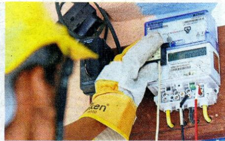
Still reliable: TNB says the smart meters are working well, with no major reading errors.
